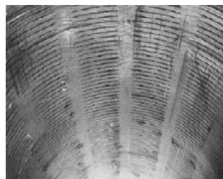
Slit filter seen from inside.
